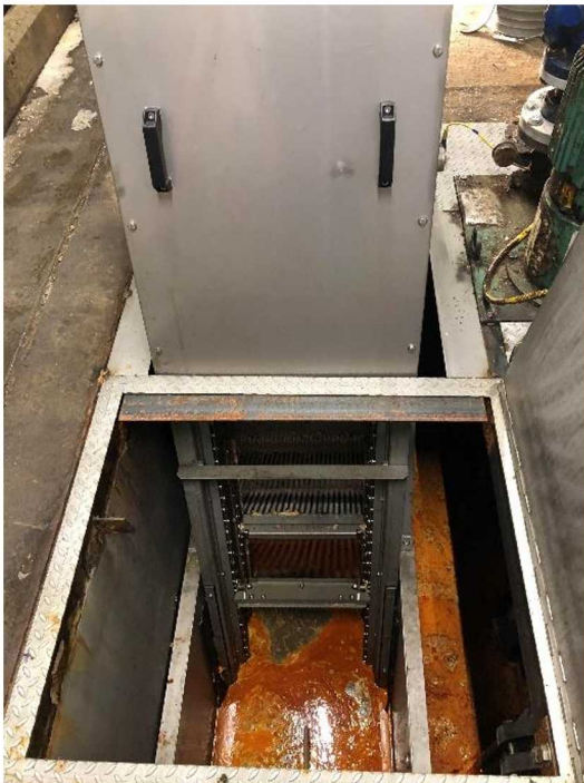
Screening at Dressing Manufacturer
