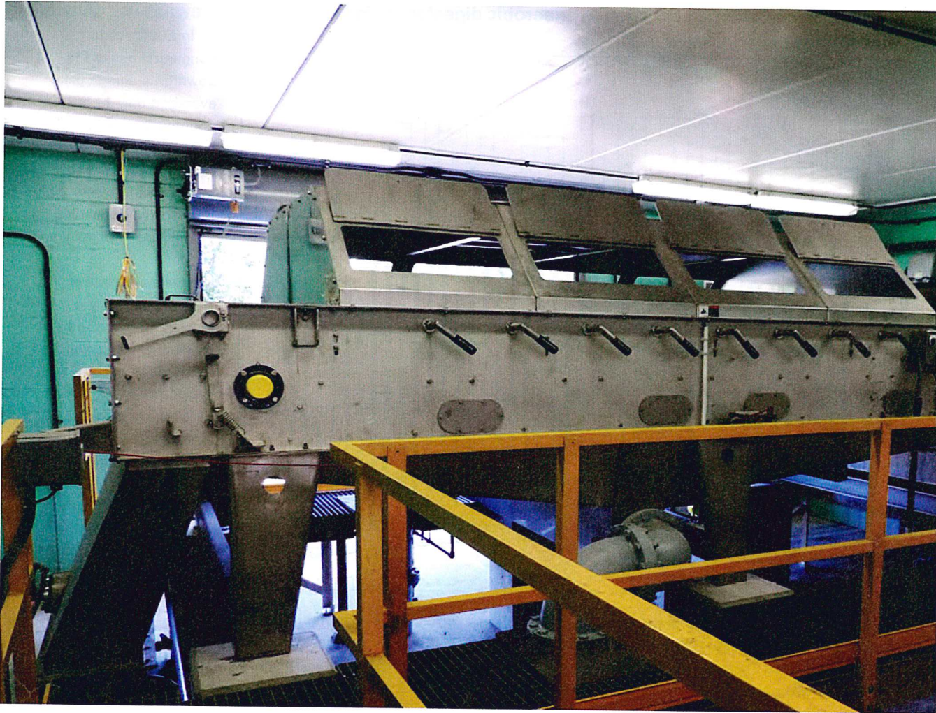
In July 2013, the city began operating two new gravity belt thickeners, which could achieve higher solids concentrations in the thickened waste activated sludge and reduce the hydraulic loading on the primary digesters. Rainbow Photographic Documentation Co. (Quakertown, Pa.)
