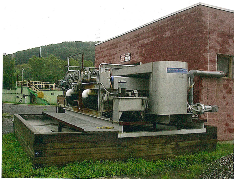
In June 2009, Bethlehem began using a temporary gravity belt thickener to replace the failing rotary drum thickener. Angela Hintz/Arcadis
