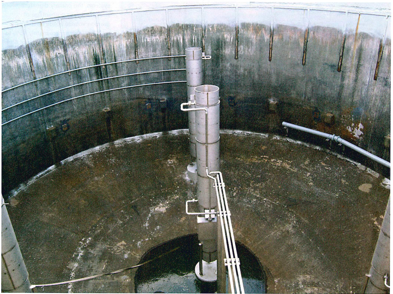
New mixing and heating systems were installed within the two existing primary digesters, helping to improve homogeneity within the solids treated by the digesters and reduce grit settlement. Rainbow Photographic Documentation Co.
