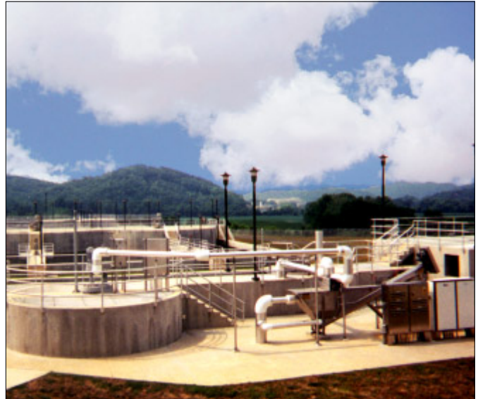
The comprehensive PISTA Grit Removal System — with stainless steel internals and components — provides the Harpeth Valley WWTP with complete system responsibility, including grit removal, pumping, washing and dewatering.
