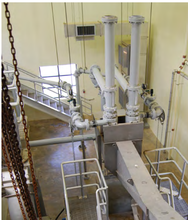
Grit trapped by the PISTA® 360™ gets moved by PISTA® Turbo Grit Pumps to the second-stage PISTA® grit washing and dewatering units.
