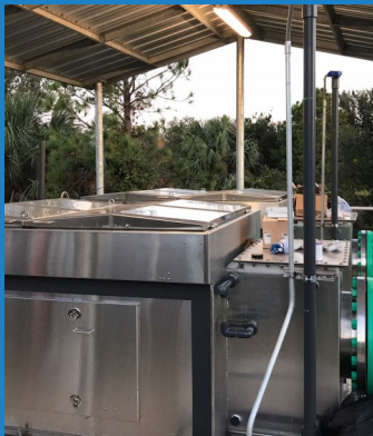
The installation at Tybee Island is simple and clean. The operators love its performance.
