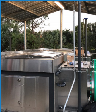
The installation at Tybee Island is simple and clean. The operators love its performance.
