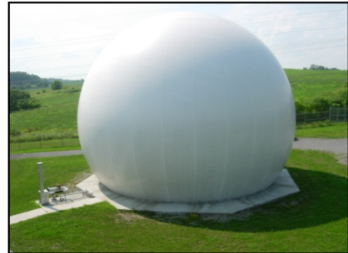
Figure 2 New JDV Double Membrane Gas Holder
