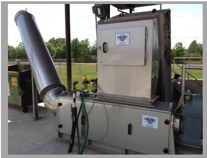
Compactor Washer Installed in Rittman
