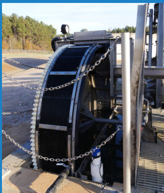
An installation at Coweta County, GA. The utility loves its performance and simplicity.
