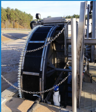
An installation at Coweta County, GA. The utility loves its performance and simplicity.
